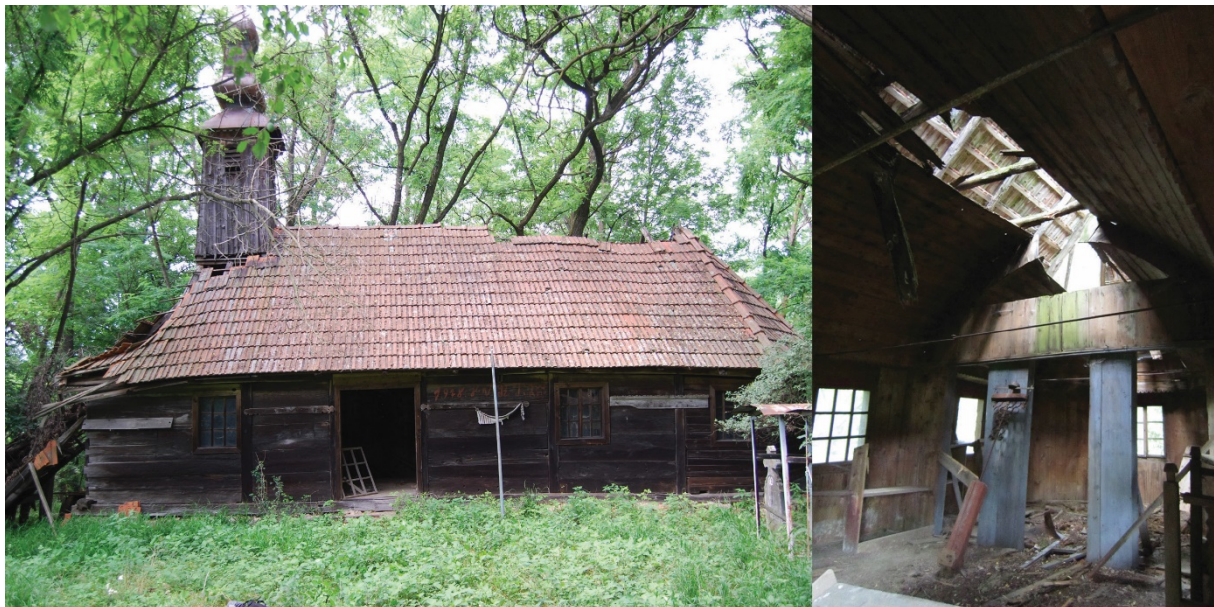
Figure 3. Pictures showing the exterior and interior in-situ condition of the wooden church of Baștea
