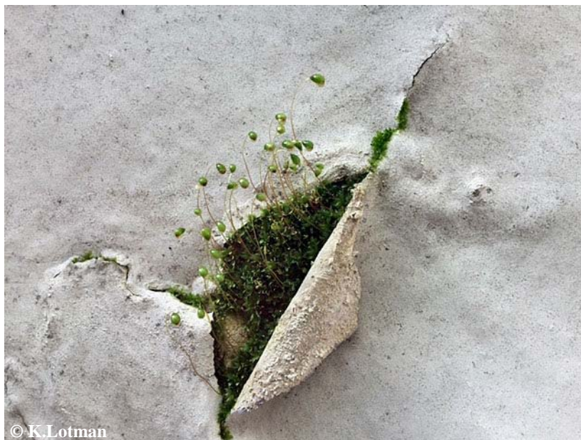
Foto 2. Harilik hellik tungib läbi mistra pragudest III korruse kabineti seinal. Funaria hygrometrica permeates through the wall tapestry „mistra“ on the second floor.
