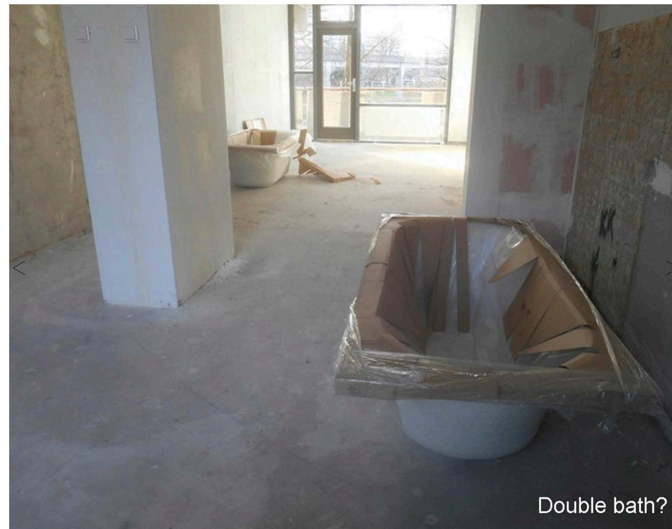
Individual choice: floor heating or radiators?
